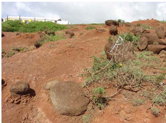
Photo 4-3: Soil erosion at Mākaha Ridge Tracking Station
